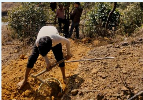
Site instruction for on-going open limestone channel (OLC) work at Laitmawsiang, Laitkroh block under MLAMP.
