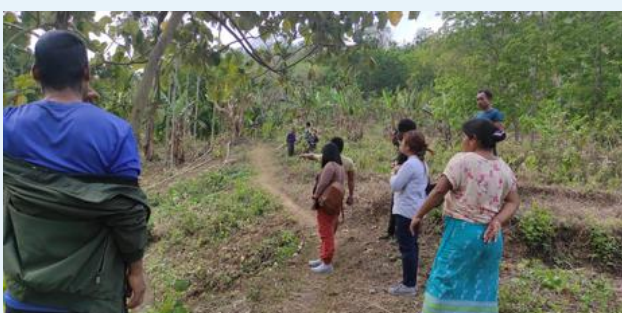
Inspection of Community Hall construction site and Community Nursery at Dokasaram Village, Redubelpara, NGH.
